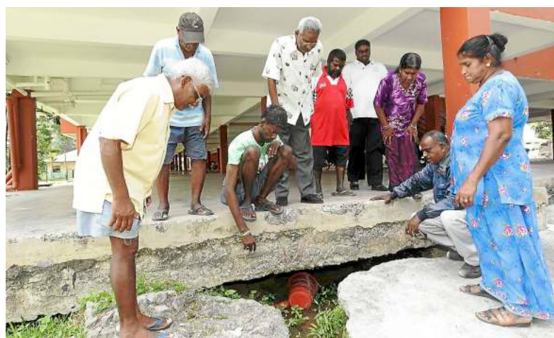
Danger below: The presence of a sinkhole leaves the flat residents uneasy.
