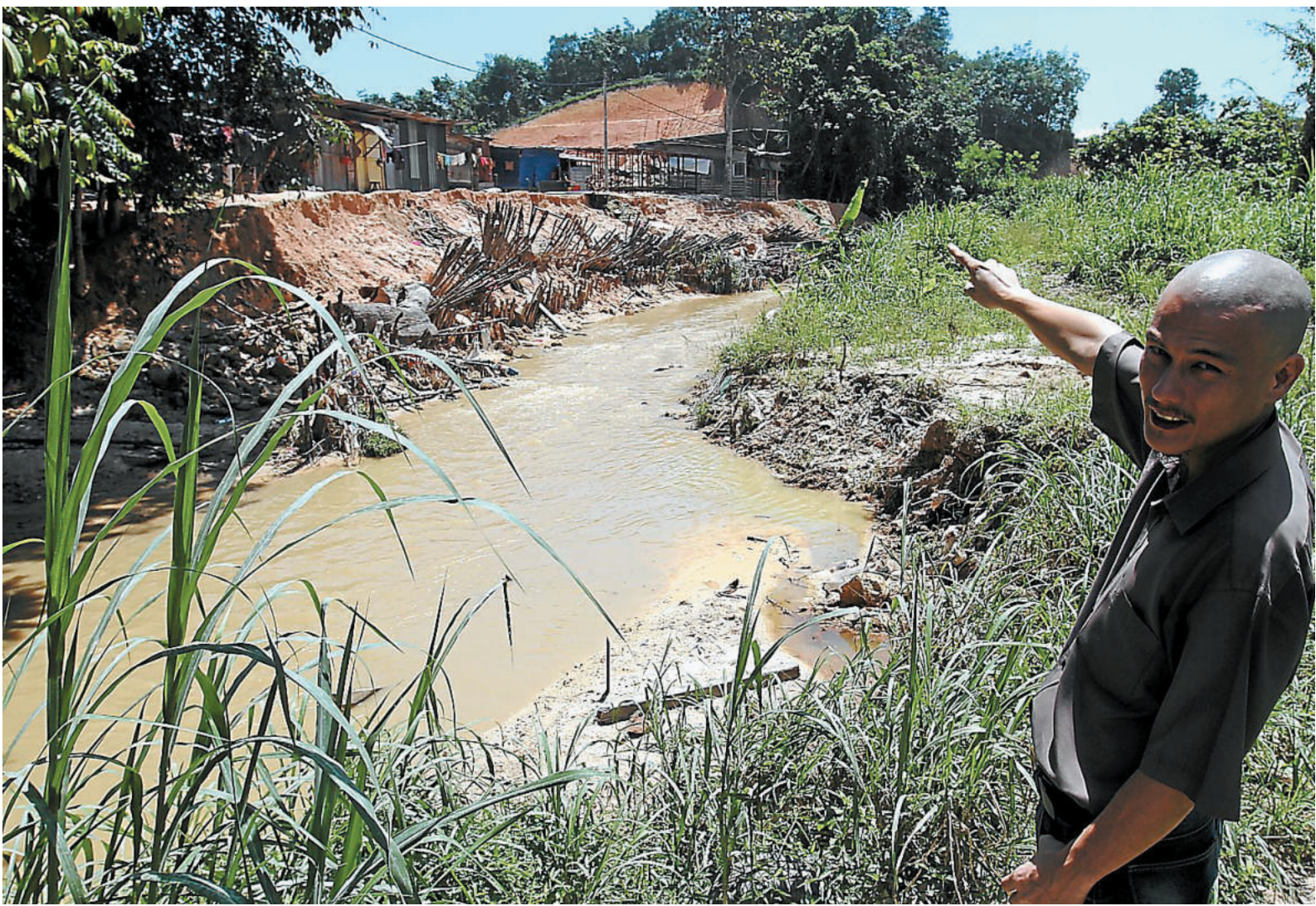
Sign of trouble: Lim pointing at the bank of a stream running through the cleared land which is on the verge of collapse.
