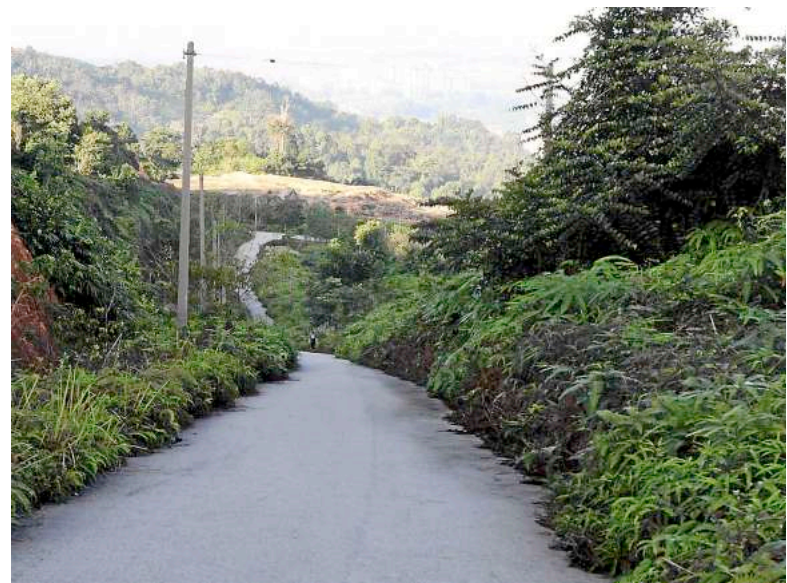
Cut off: The cables for the electricity poles erected all over Bukit Enggang have all been stolen.
