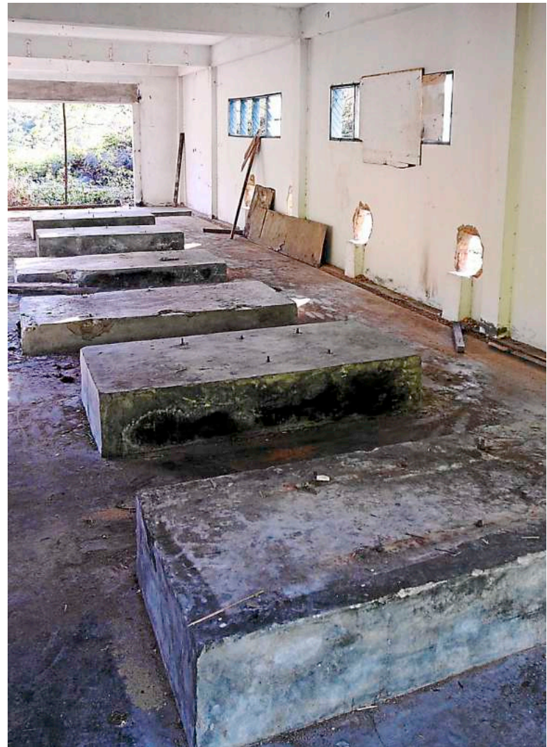
Bleak outlook: An abandoned utility building inside Bukit Enggang.
