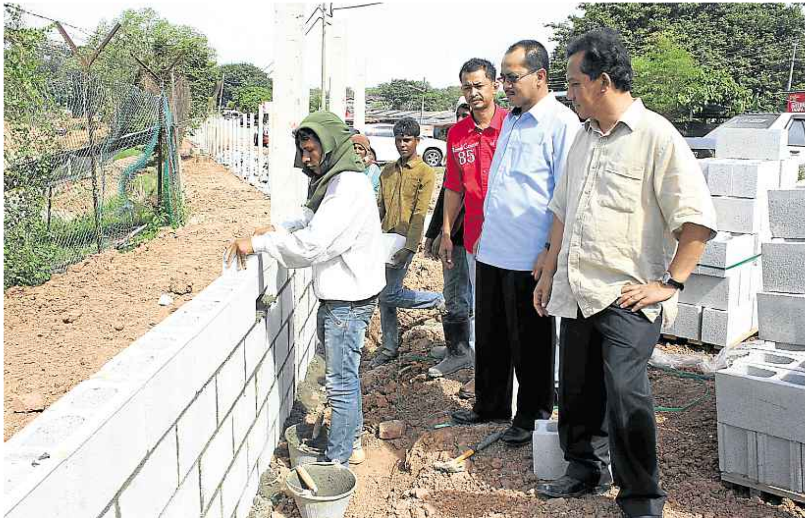
Cergasjaya Properties Sdn Bhd director Ahmad Shaker Ahmad (right) and Zulfitri Yaakob (second from right) inspecting the progress of the concrete wall to curb smuggling activities near the Bukit Kayu Hitam Duty Free Complex in Kedah. Pic by Rahmat Othman
