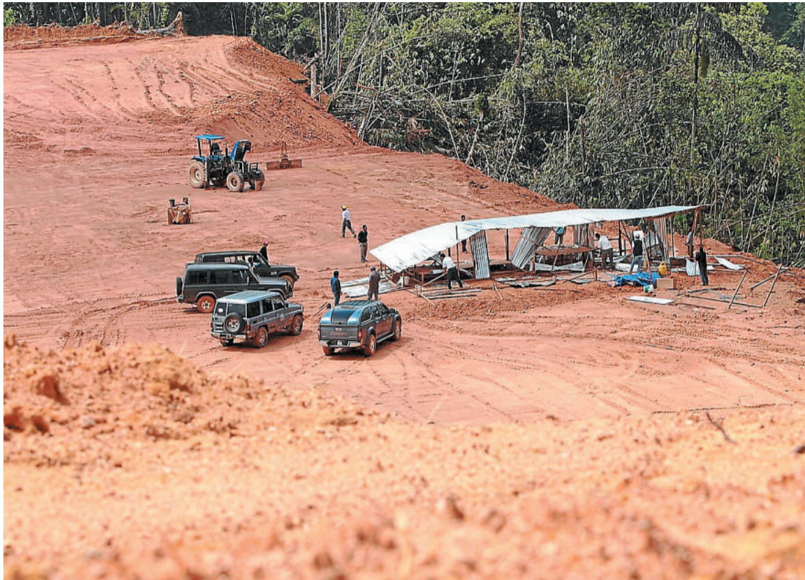
Torn down: Enforcement officers destroying newly built workers' quarters on illegally cleared land in Pos Terisu.
